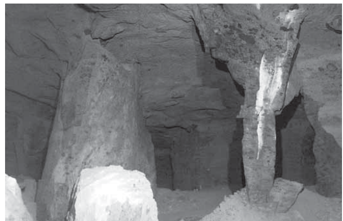
Fig. 17 Internal view of a trachyte mine (Del Prete, 2004) at the foot of Camaldoli hill (Napoli): huge rocks detached from the vault and from the pillars (photo: S. Del Prete). The pillars are evidently compressed by the static solicitations of the loads.
